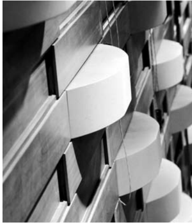
Figure 2.2 Application of optimized curved diffusers (OptiCurve™) in the Hummingbird Centre, Toronto. (Consultant: John O’Keefe, Aercoustics Engineering Ltd.; after D’Antonio and Cox 1 .)
